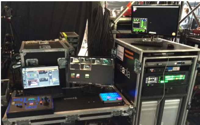
The control room during the tour
